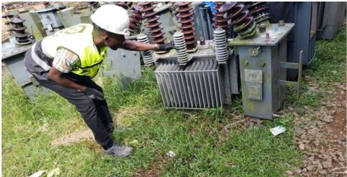
Figure 4: surge arrester of a three phase distribution transformer
